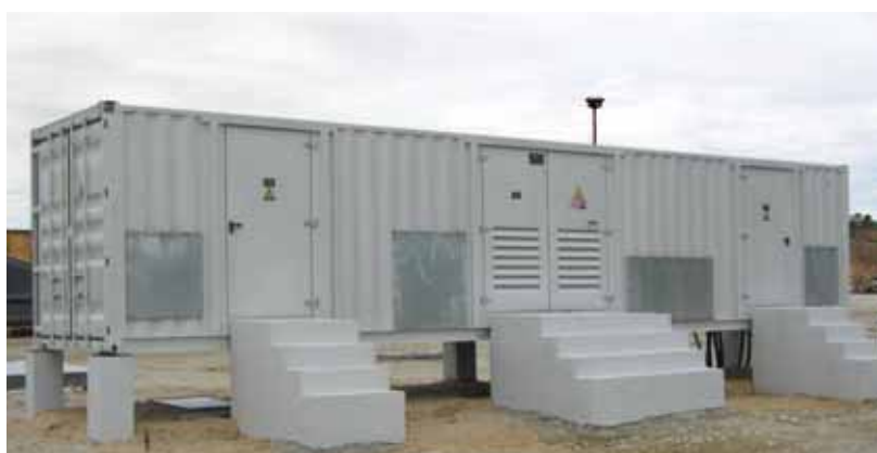
Cabine containerizzate, i locali ideali per i nuovi quadri Minifluor XS Small containerized substations are the ideal location for the new Minifluor XS switchboards.
