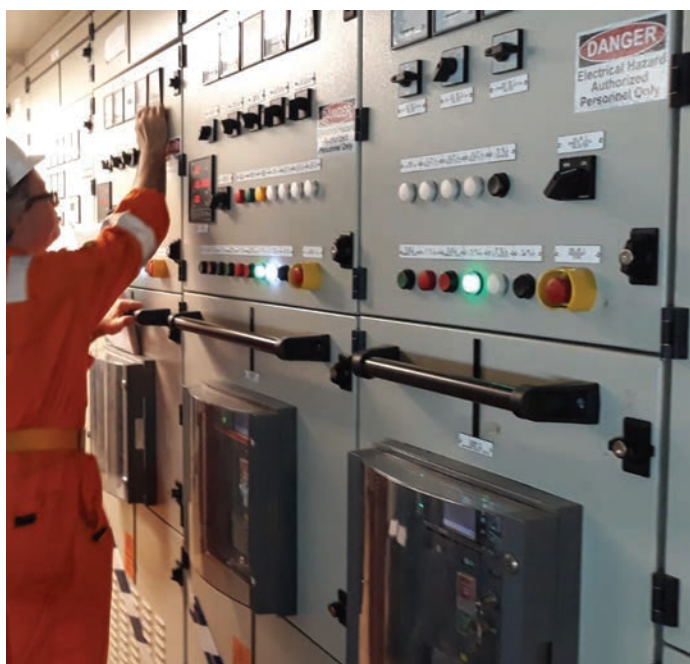
I quadri per la Liza Destiny / Switchboards for Liza Destiny
