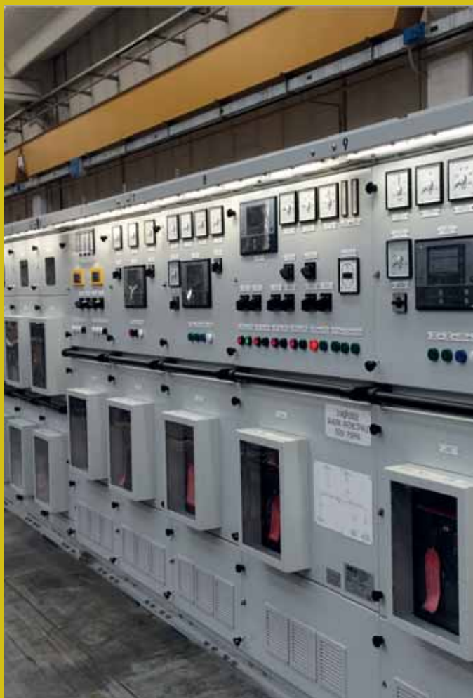
In alto, rendering della nave Landing Helicopter Dock (LHD) Qui sopra, i quadri realizzati per il progetto PPA / In the top picture the rendering of the Landing Helicopter Dock (LHD) ship. Above the switchboards produced for the PPA project
