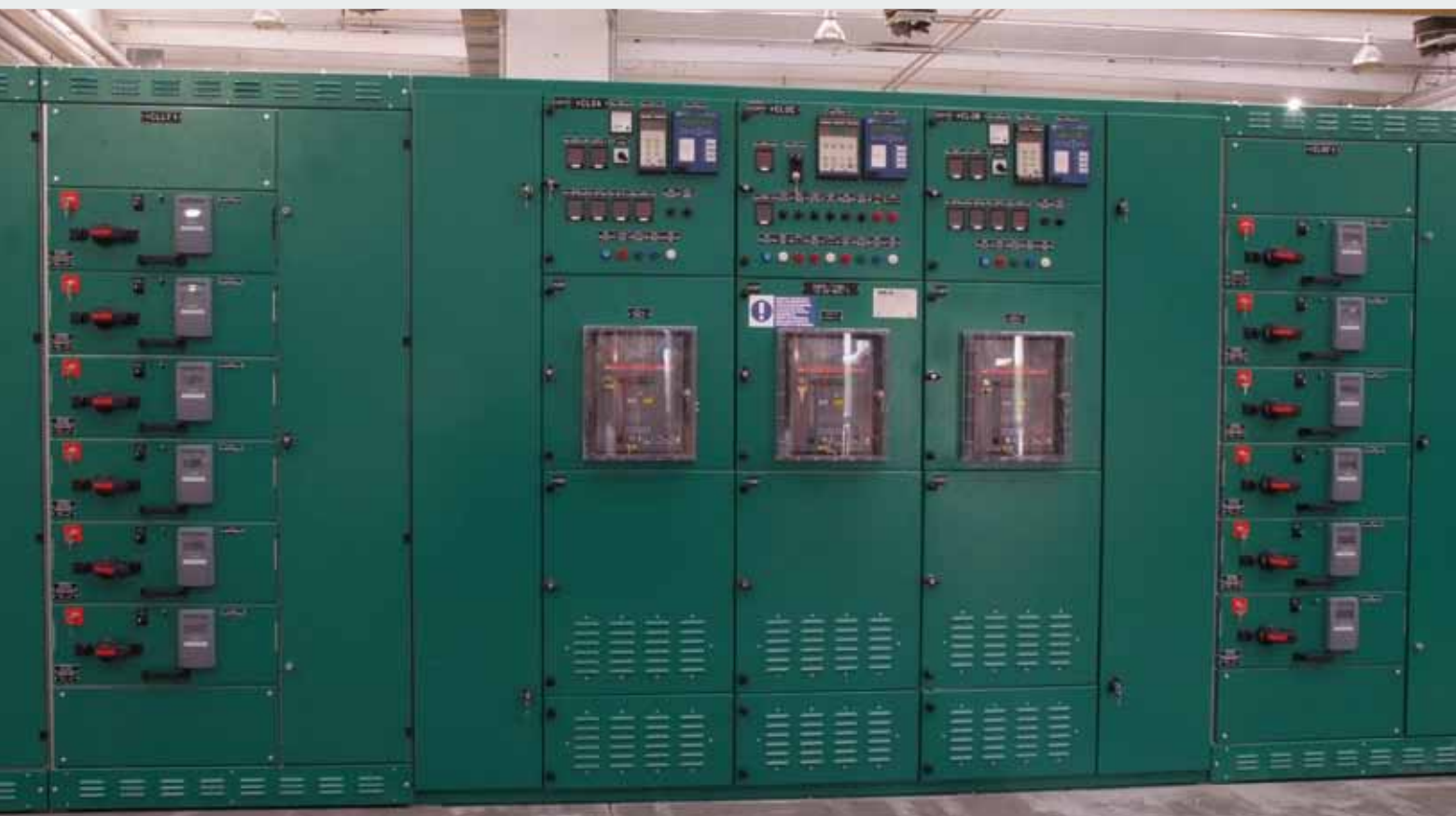
Quadro elettrico Power/Motor control center - RandPower/Motor control center switchboard
