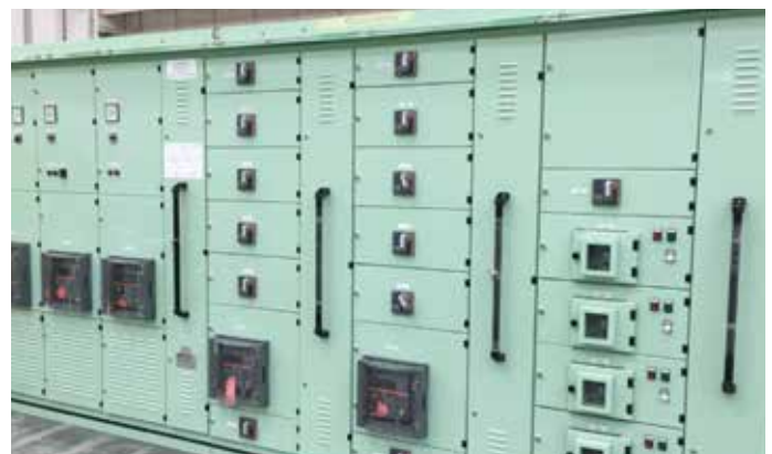
Virgin Voyages Fincantieri Shipyard - Main LV Substation 690V - 2500A - 50kA
