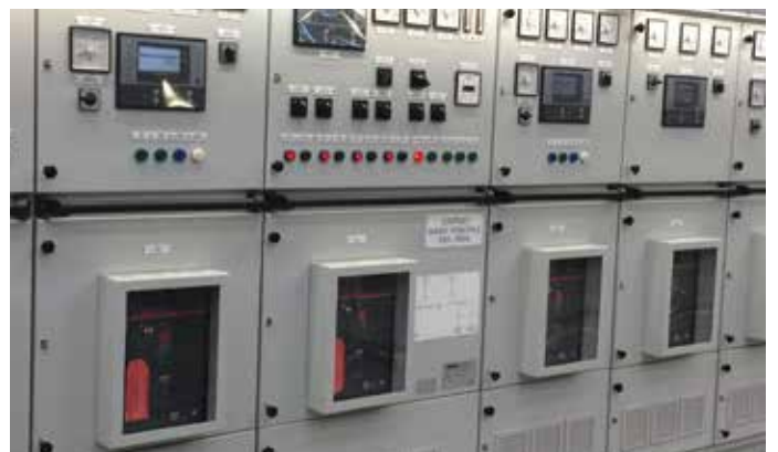
LV Main Switchboards with Shock Withstand Requirement 690V - 4000A - 65kA PPA - Italian Navy
