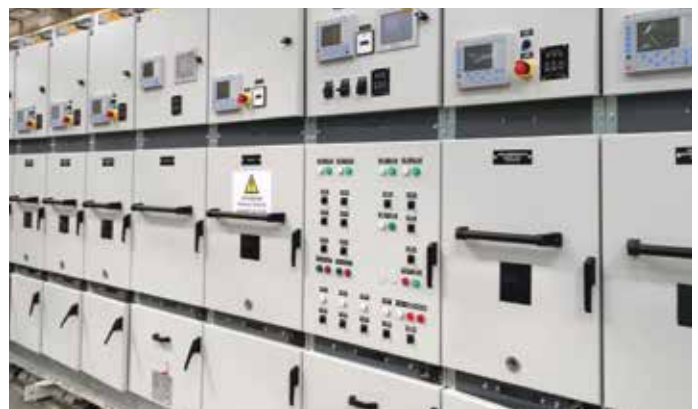
MV Main Switchboard with Shock Withstand Requirements 12kV - 630A - 31,5kA LHD - Italian Navy
